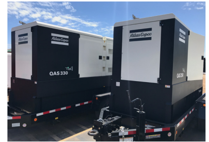
Portable & Standby Generators
